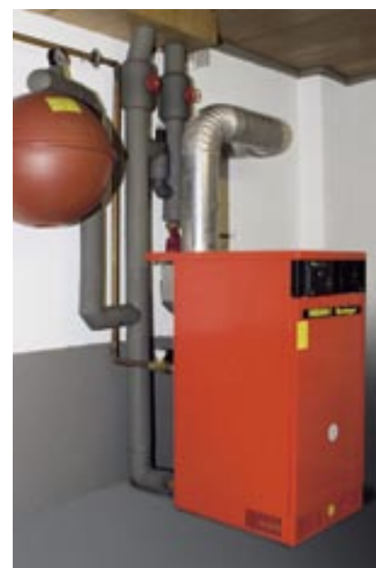
Even in modern, well-insulated houses further energy savings can be achieved by insulating heating and hot water systems professionally
