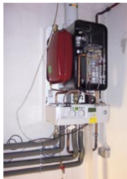
Optimal insulation can greatly reduce heat losses from pipes
